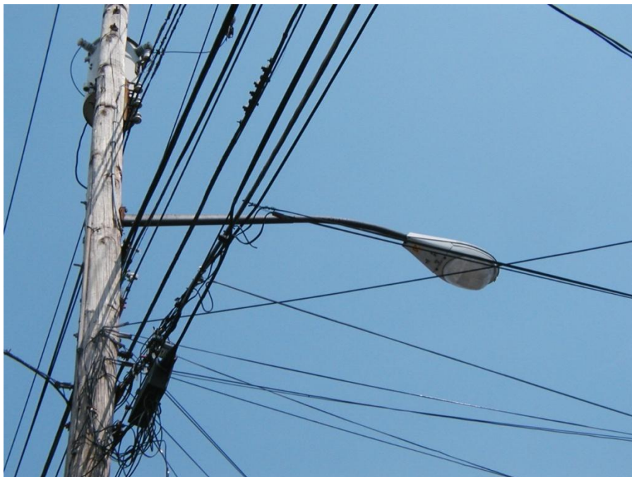
Figure 7. Typical HPS Streetlight Placement [12]
